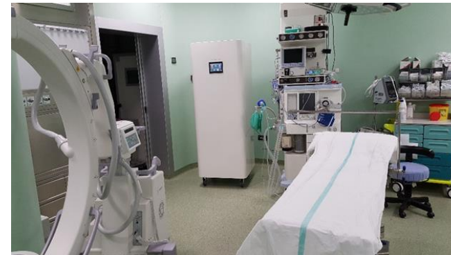
JONIX mate sanitizing and filtering cabinets placed in two hospital's operating rooms in Calabria where the test was carried out
